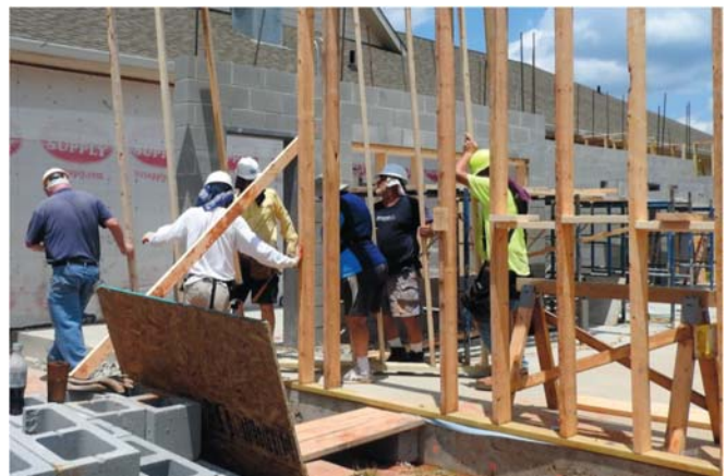
Above, laborers raise a wall at Christ Lutheran Church in Perry, Ga. as part of its expansion to add classrooms and a fellowship hall.
